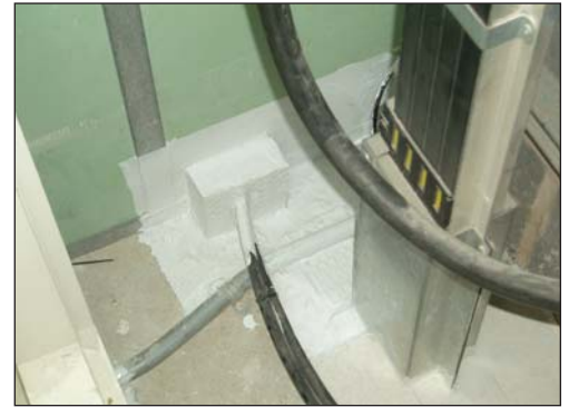
RISER CUPBOARD AFTER
