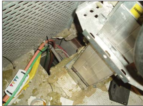
RISER CUPBOARD BEFORE
